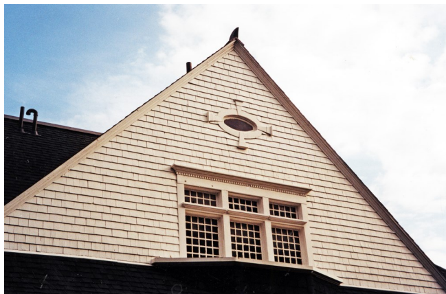
The three mullion-paned windows and oculus that illuminate only an unused attic
