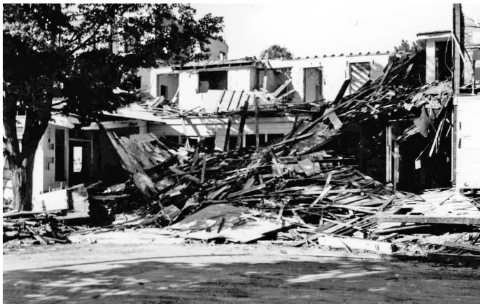
Entryway filled with fallen lumber
